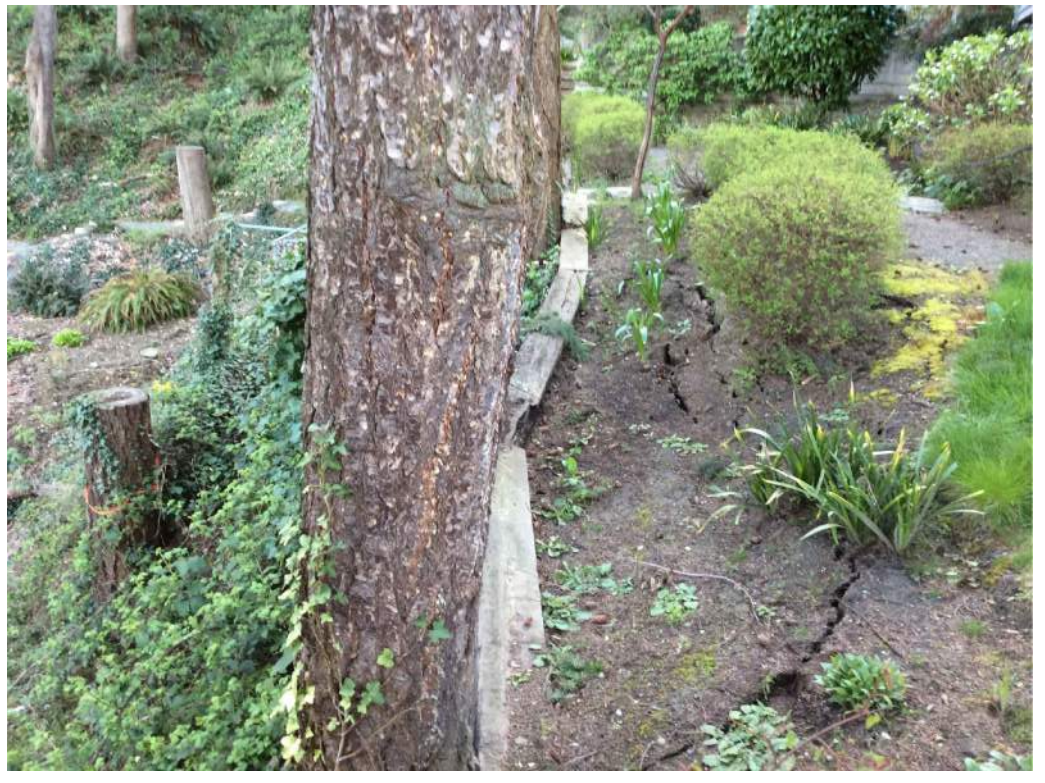
VISIBLE FAILURE OF SLOPE
