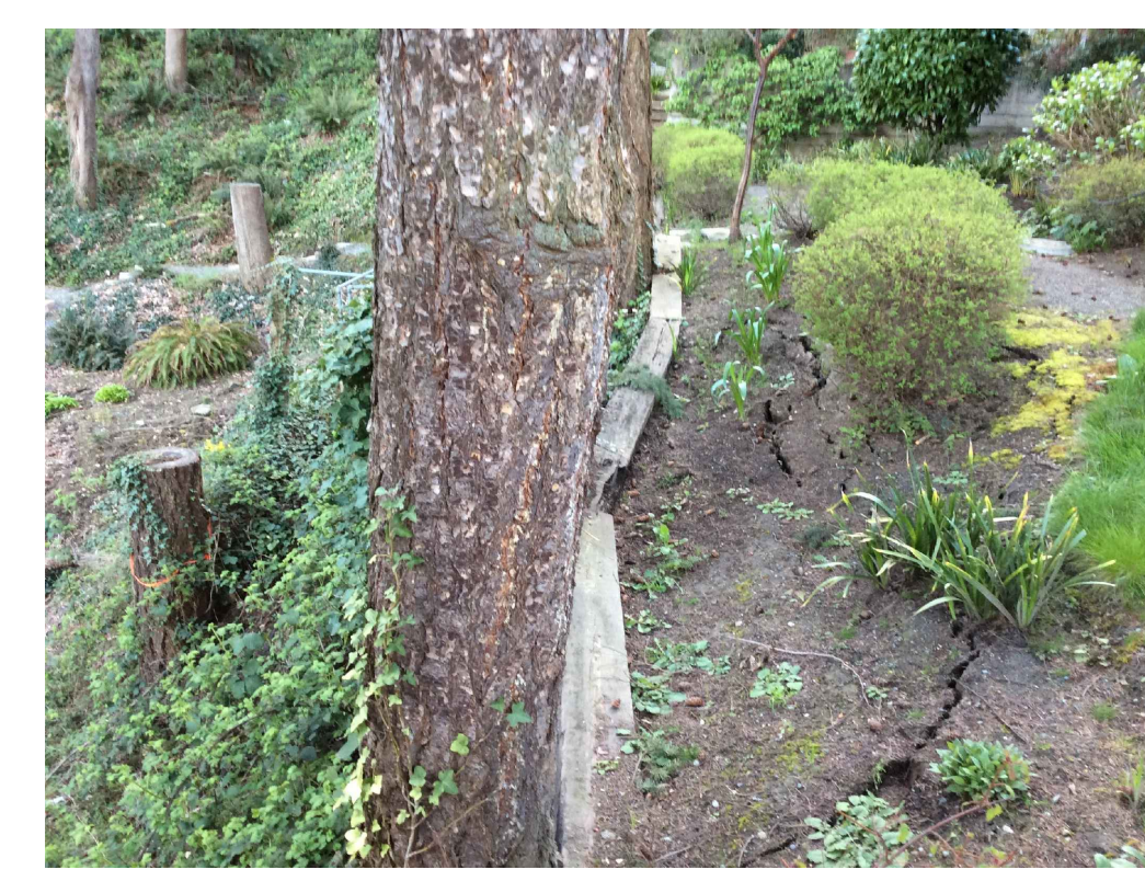
VISIBLE FAILURE OF SLOPE
