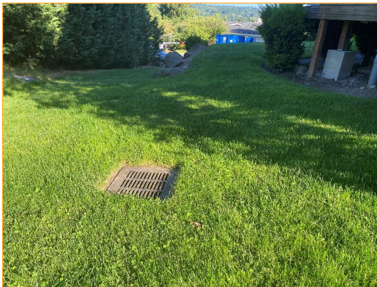
Photo 2 – Facing southwest along the southwestern portion of the property. Runoff sheet flows to a privately owned catch basin within the storm drainage easement and continues southeast.
