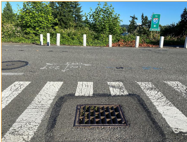
Photo 6 – Facing southeast along the west side of E Mercer Way. Runoff is collected by a catch basin and continues southeast through a tennis court.
