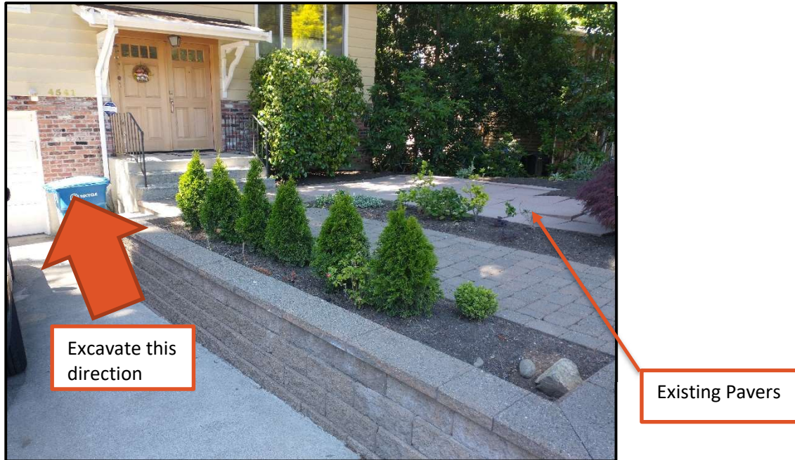
Photo 4. Front entry of the home viewed from the east. I recommend that excavation begin from the existing structure to the new foundation area to protect the newly exposed soil. The existing pavers should be removed by hand and the TPZ fencing should be placed.
