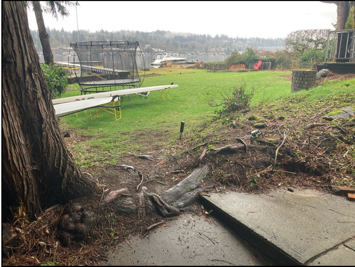
Photograph 4. Tree 79, a 29-inch western redcedar with significant root conflicts with the patio and concrete path. This is the only large tree currently proposed for removal.
