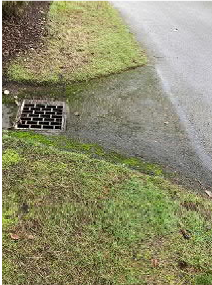
Picture 9: ROW in front of 2203 70 th Avenue SE CHANGE TO 18" AT THIS CB
