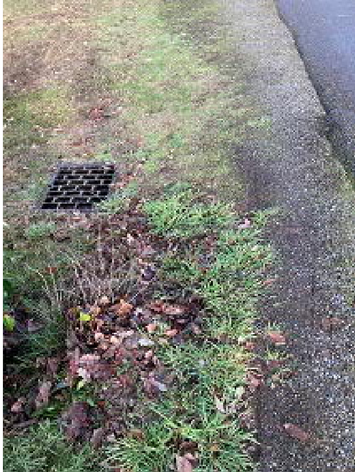
Picture 1: ROW in front of 2251/ 2243 71 st Avenue SE Water flows north (toward the top of the page)
