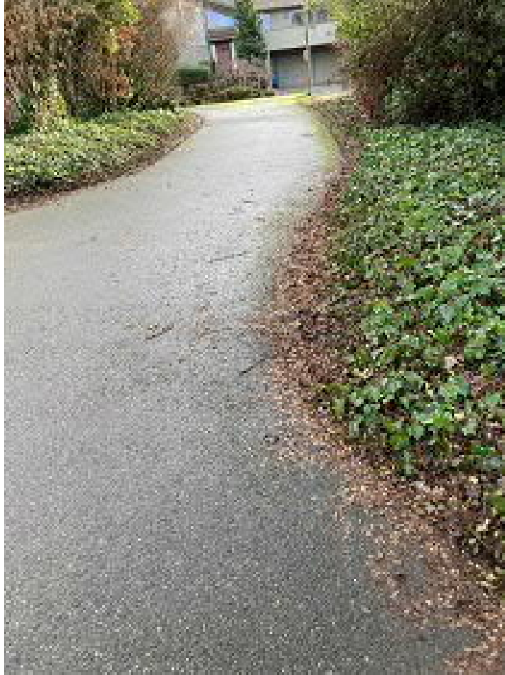
Picture 11: Aubrey Davis Park looking SE toward 2212 66 th Avenue SE The catch basin is under the ivy somewhere near here 18" SD WSDOT OWNED PIPE
