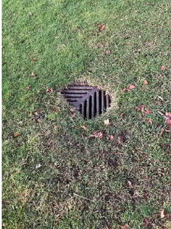
Picture 13: Aubrey Davis Park at a low point near the playground From here the storm pipe goes west toward W. Mercer Way 18" SD WSDOT OWNED PIPE
