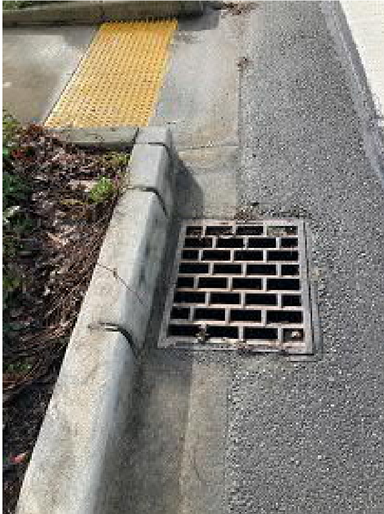
Picture 15: West Mercer Way 18" pipes head south under W. Mercer Way 18" SD WSDOT OWNED PIPE
