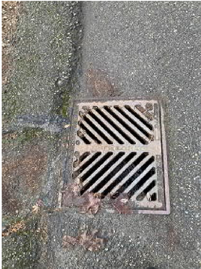
Picture 8: Southeast corner of SE 22 nd Street and 70 th Avenue SE From here, storm pipe crossed west under 70 th Avenue SE 12" SD
