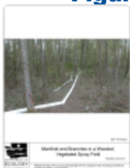
Figure II-3.25: Manifold and Branches in a Wooded, Vegetated Spray Field
