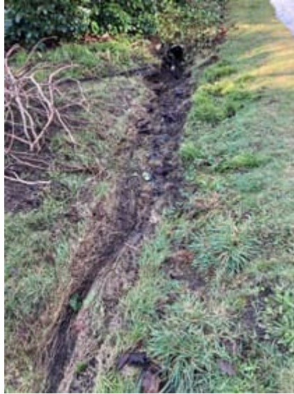
Picture 5: South ROW in front of 7103 SE 32 nd Street garden; looking west (downstream)
