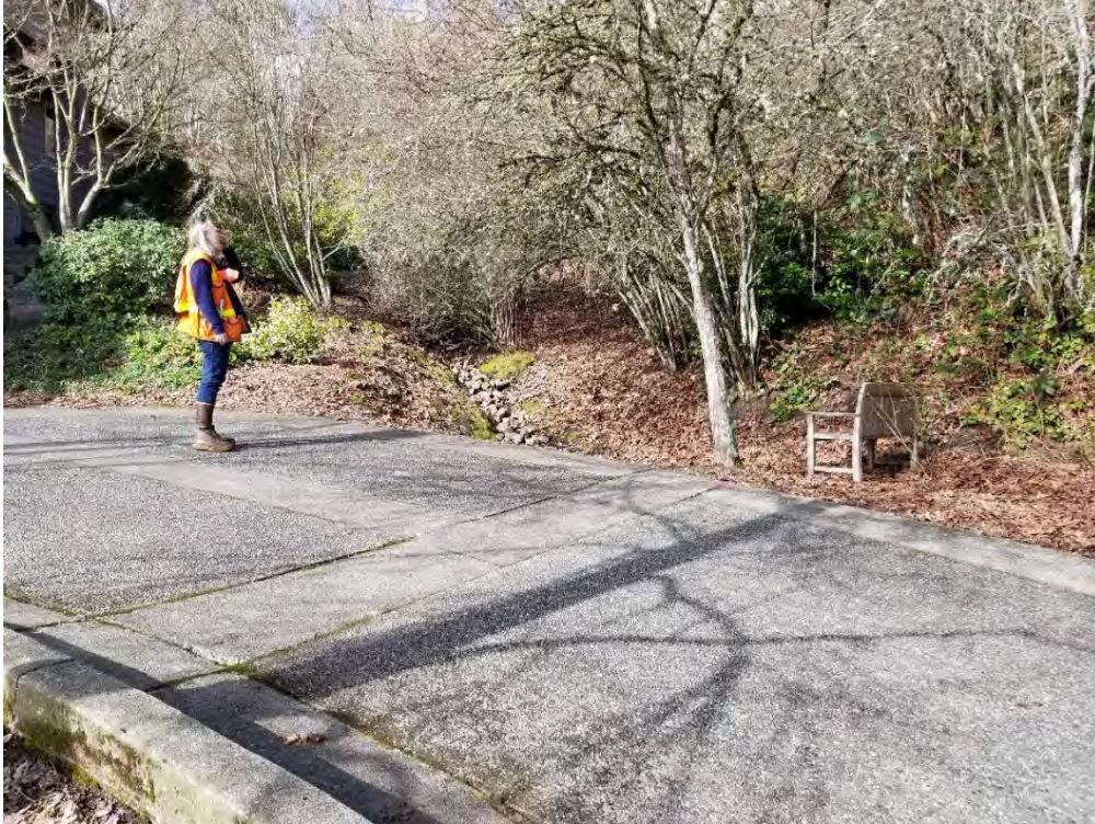
Photo 11—Driveway to 7511 92 nd Avenue Southeast. The stream channel is conveyed under this driveway by a culvert.
