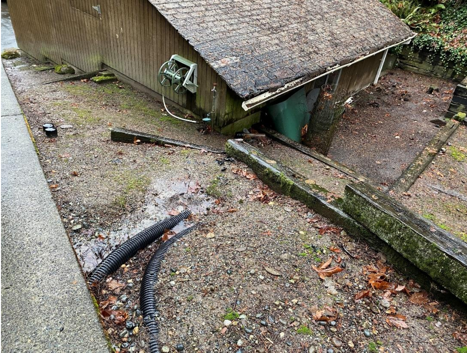
At driveway, looking Southeast toward existing garage. Disconnected subsurface pipes along south side of driveway
