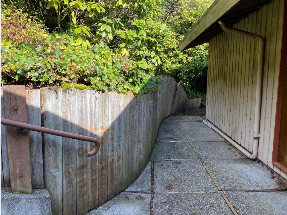
Yielding timber retaining walls at along east toe of slope.
