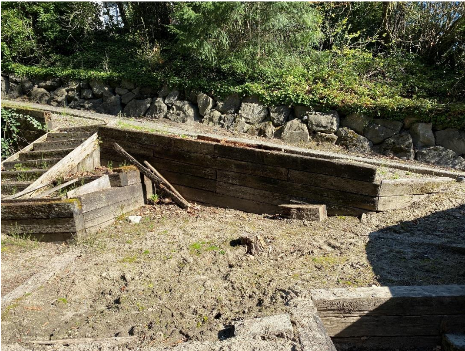
View from west of garage, looking north. Yielding timber retaining wall south of driveway
