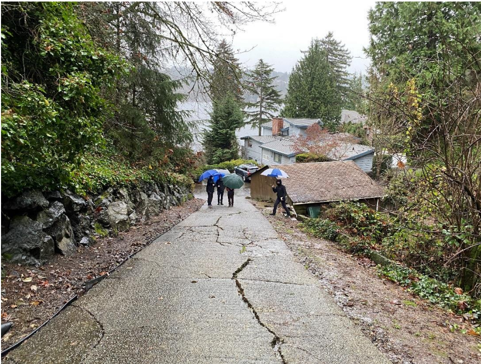
Looking east, down the driveway. Existing garage at the right. Visible cracking of concrete driveway.
