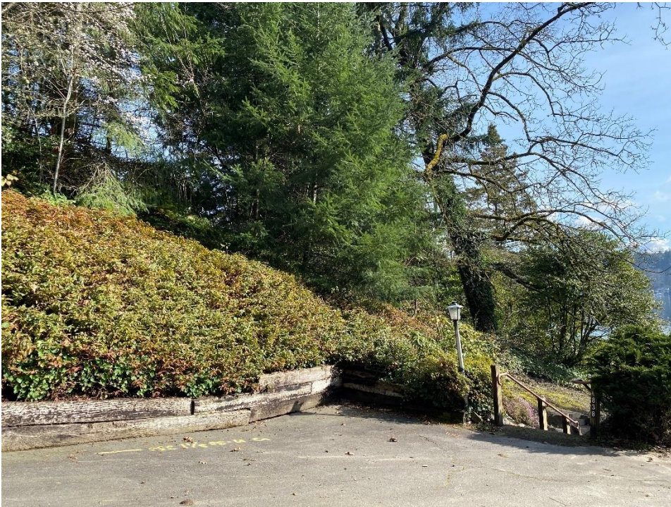
Yielding timber retaining wall north of the parking pad. Existing stairs at right.
