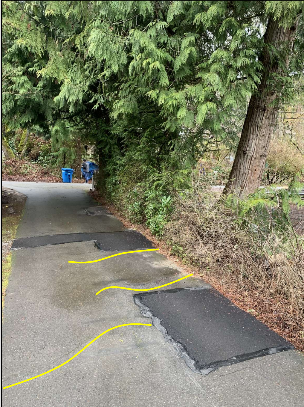
Photo 2. Exceptional tree D is on the right and trees E and F are a part of the hedgerow to the left. These trees are offsite but growing close to the driveway to the house. There is cracking in the hardscape (outlined by yellow) suggesting these trees have structural roots close to the surface under the hardscape. Plans do not call for the removal or replacemen of these trees.
