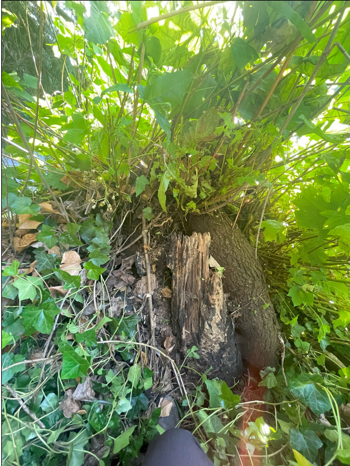
Photo 7. Base of Tree #14. Eastern trunk failed and remaining western trunk over Island Crest Way was cut. Decay-causing fungi Kretzschmaria deusta was present.
